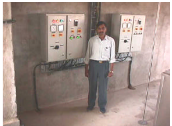
Power Control Panel
